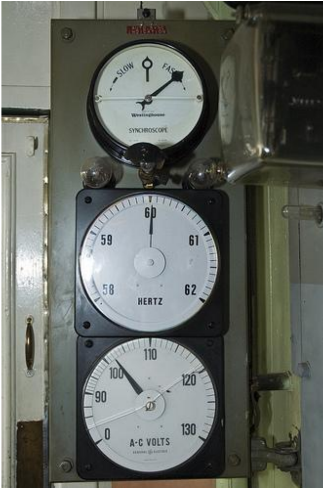
Fig 2. Control panel showing the synchroscope (top), hertz meter (middle), and voltage meter (bottom) at the Boulder Canyon Hydroelectric facility.
