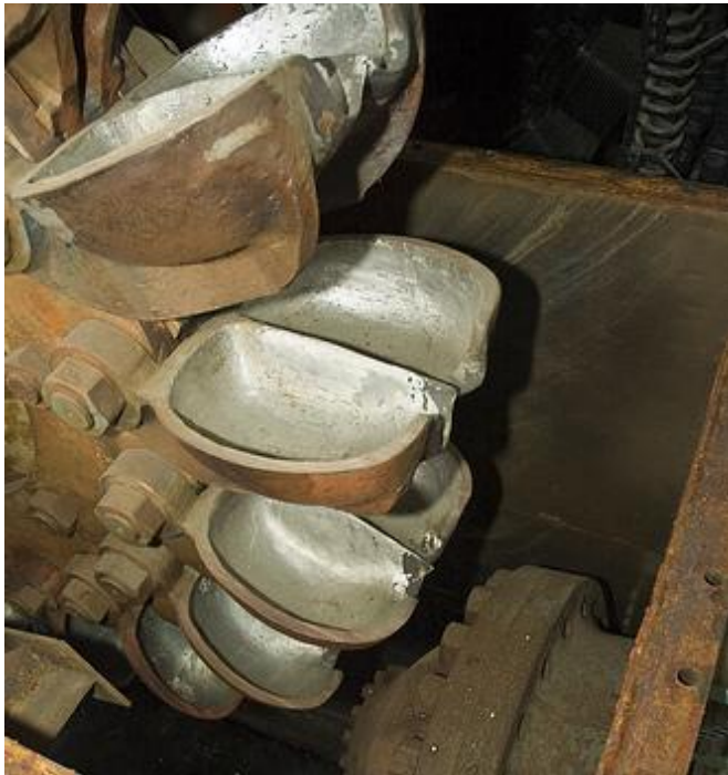
Fig 5. Buckets on the "A" Pelton wheel at Boulder Canyon Hydroelectric facility.
