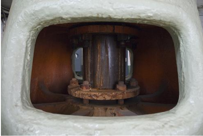
Fig 4. Piston that controls water flow at the end of the penstock at Boulder Canyon Hydroelectric facility.
