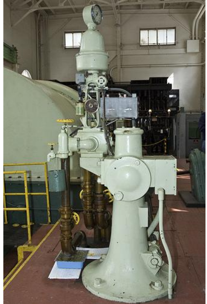
Fig 3. Synchroscope for generator "B" at Boulder Canyon Hydroelectric facility.
