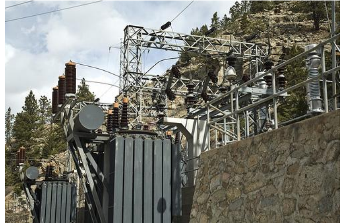
Fig 6. Switchyard next to Boulder Canyon Hydroelectric. The two 12.5 kVA; 115kV Wye/ 4kV Delta transformers can be seen near the bottom left quadrant.
